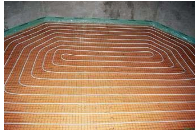
Central Heating pipes Underneath a parquet
